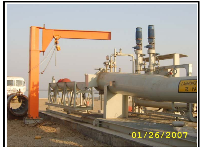
설치된 PIGGING SYSTEM
